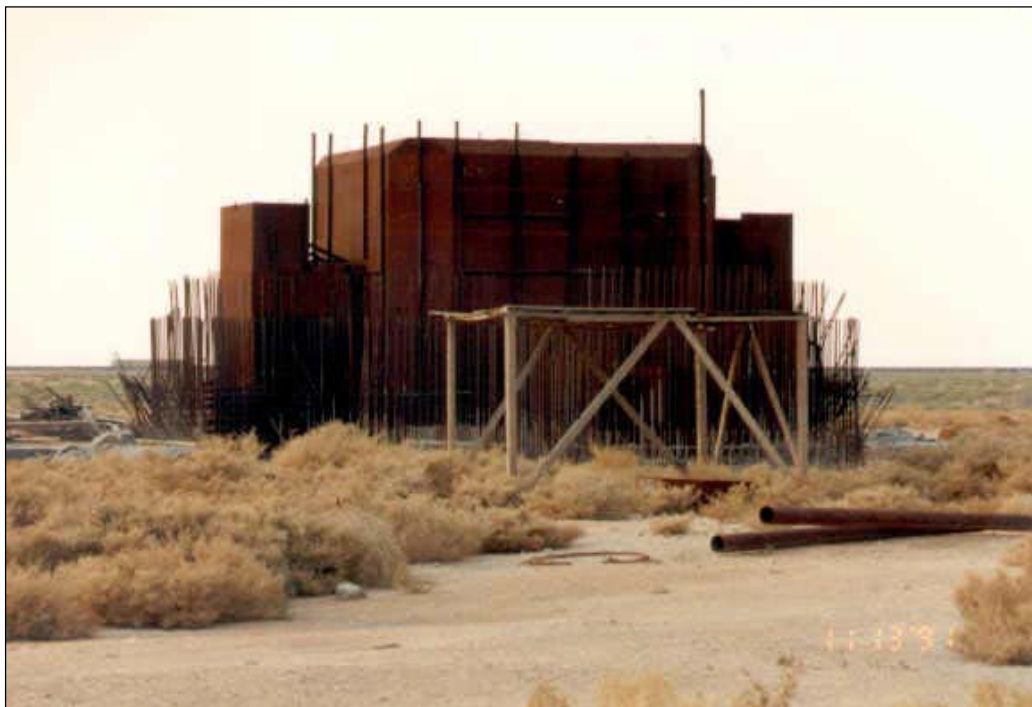
Figure 4. Building for testing polonium-beryllium neutron initiators at al Atheer. 1991. Los Alamos National Laboratory
